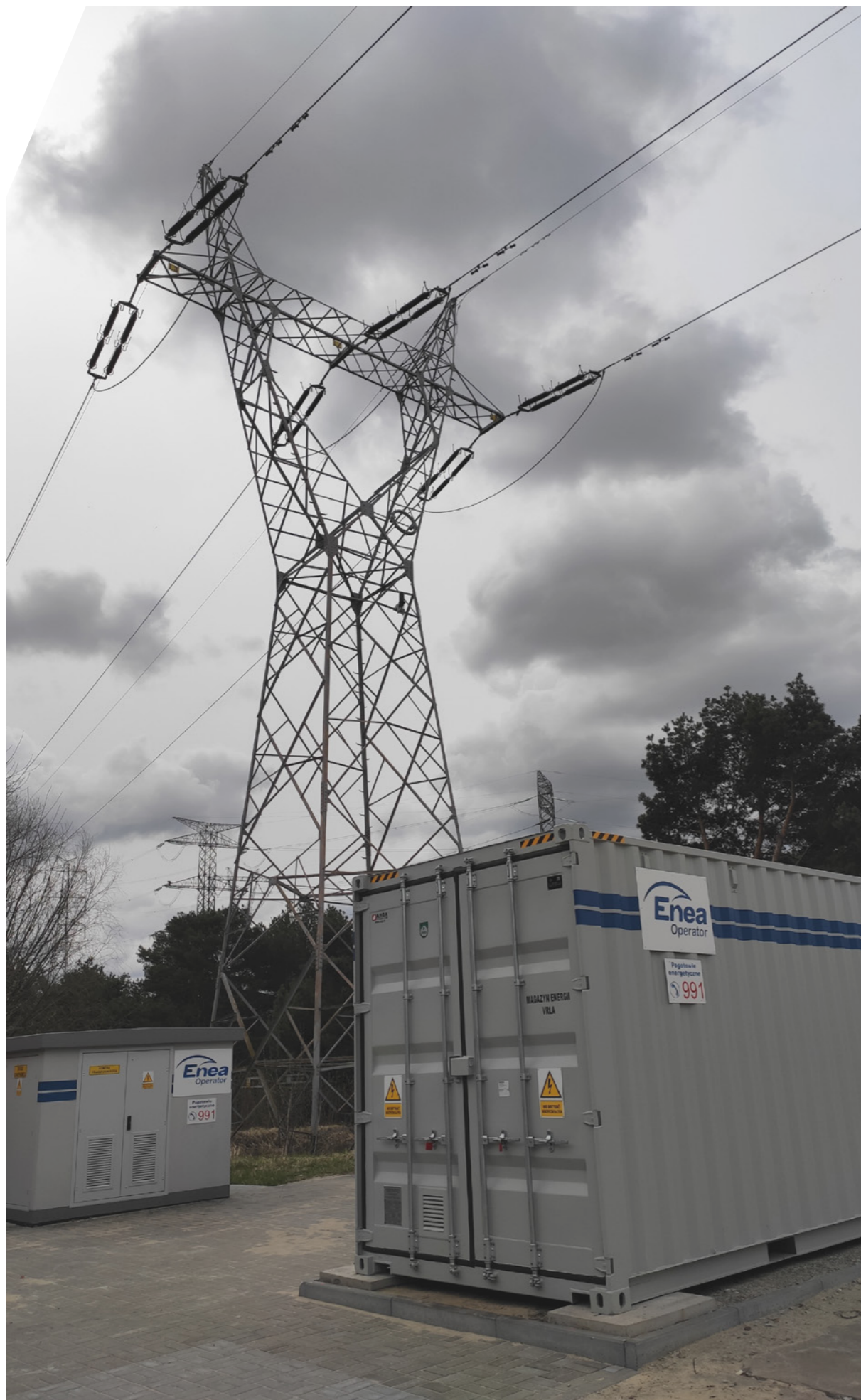
Enea Operator, Magazyn energii
